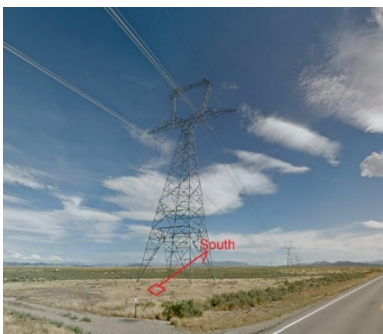
< 500 KV DC Transmission Lines and Tower
